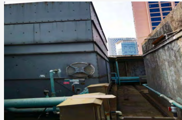
High-Energy consumption cooling tower before transformation
